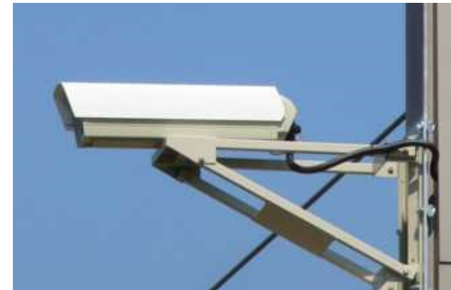
The Uplift sensor is mounted on a portal.
