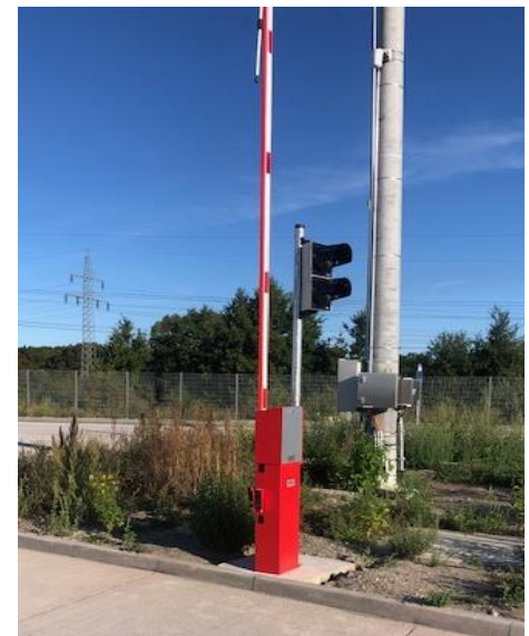
Picture 3: Barrier system incl. intercom
