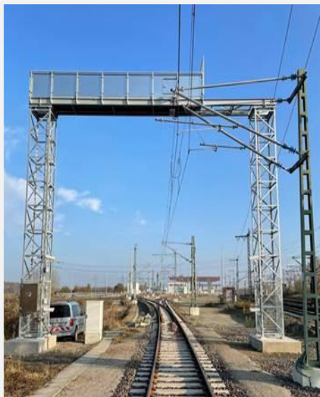
Picture 1: Rail Gate, walk-in portal
